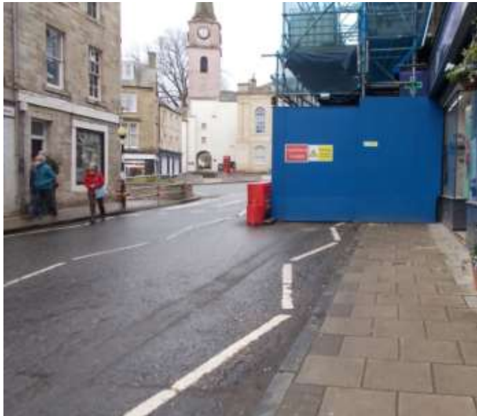
Termination of footway on High Street.
